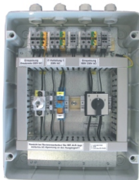
Bypass - BSV Kompakt
